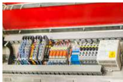
Advanced, PLC based control and DAQ electronics
